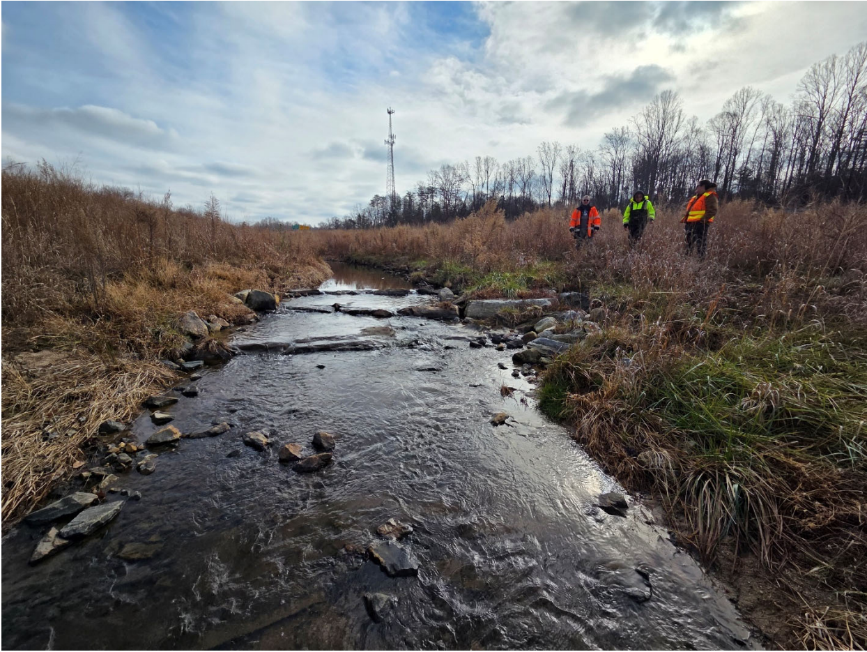
Supplemental Photo: Upstream view @ Sta. 19+25; left bank erosion, stream piping under mid-rock and roll riffle sill end
